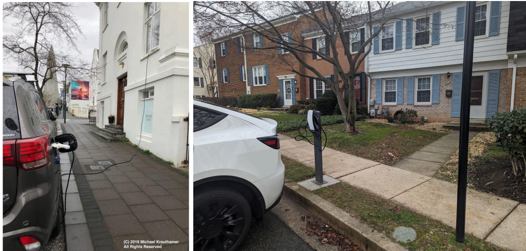
Motivation for DC cord cover guidance (at left). Rockshire Townhome EV charging in assigned parking spaces (at right).
